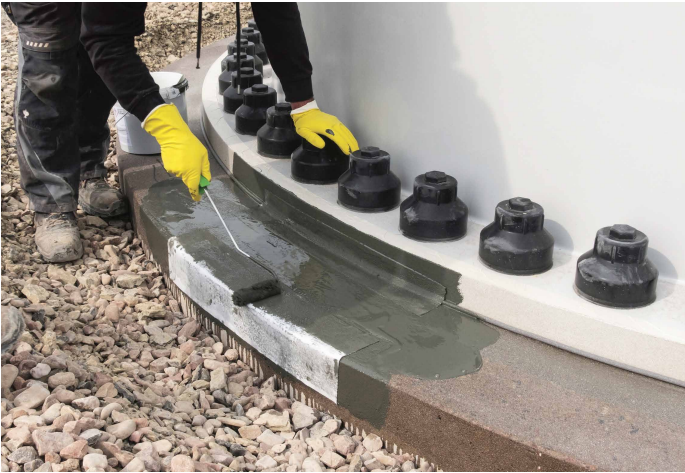
Applying a second layer of KEMPEROL to the edge of the base.
