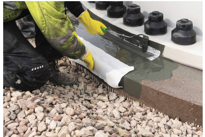
Working the fleece into the KEMPEROL layer at the edge of the base.
