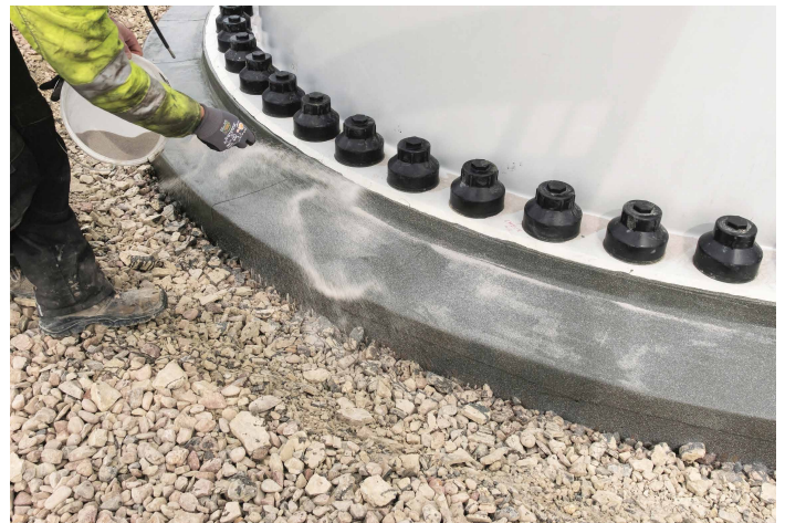
Scattering the waterproofing with KEMCO NQ 0408 Natural Quartz . (Please only scatter up to 10 cm away from the joint).
